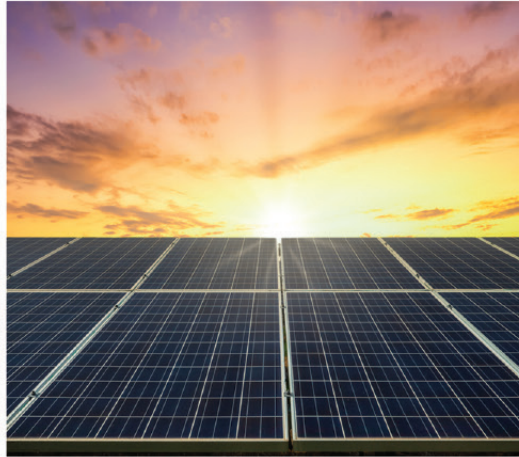
Rooftop Solar PV Systems
